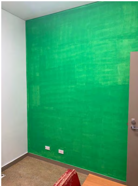
First coat of paint on our greenscreen wall in the mini-broadcasting studio. This is about the stage we had reached at the end of 2020/21 but by the time of our AGM you can now see the room in a finished state.
